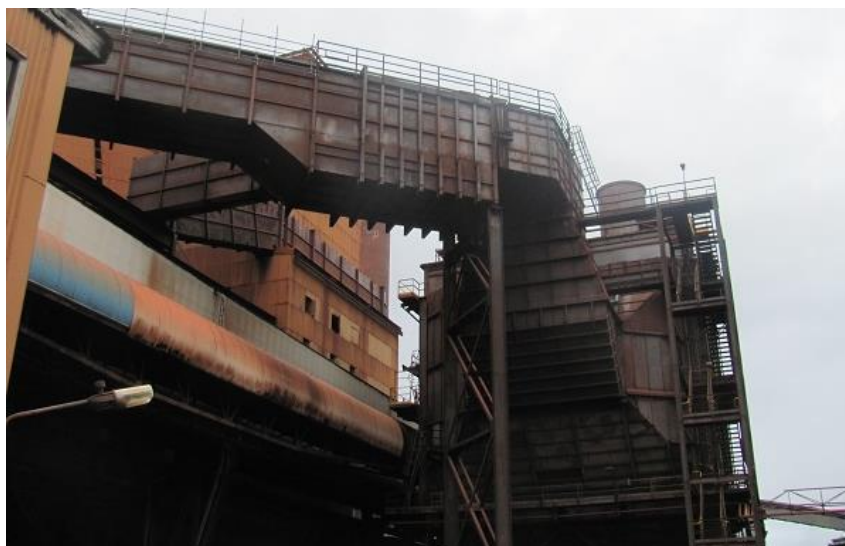
Photograph 4 Sinter Machine Room Dedusting (Duct and Precipitators in Foreground and Stack in Background) (24 February 2019)
