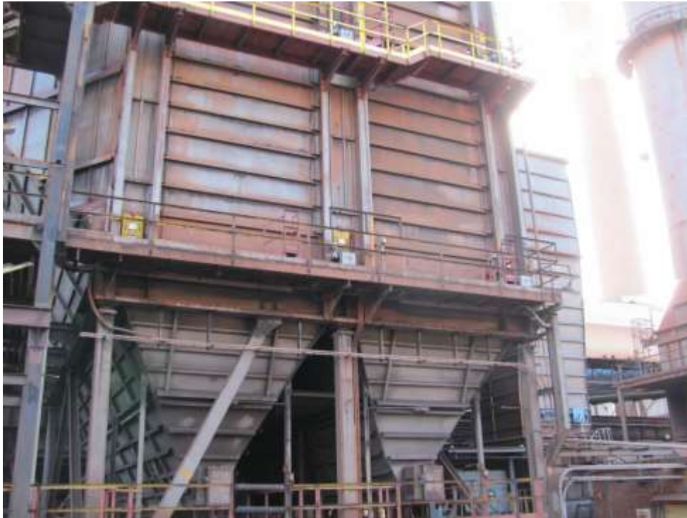
Photograph 5 Precipitators for Sinter Machine Room Dedusting System (24 March 2016)
