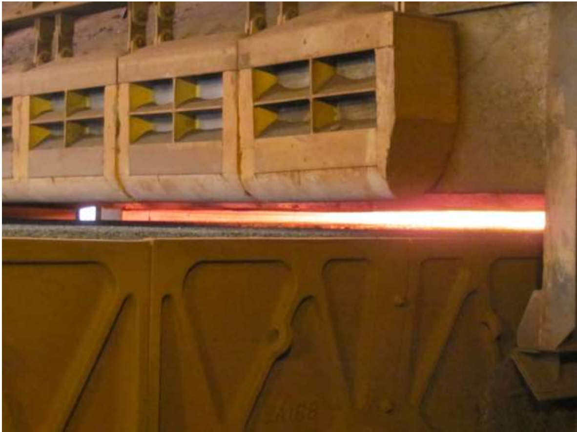
Photograph 3 Ignition Furnace (24 March 2016)
